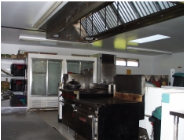
An exhaust hood vents fumes from cooking surfaces.
