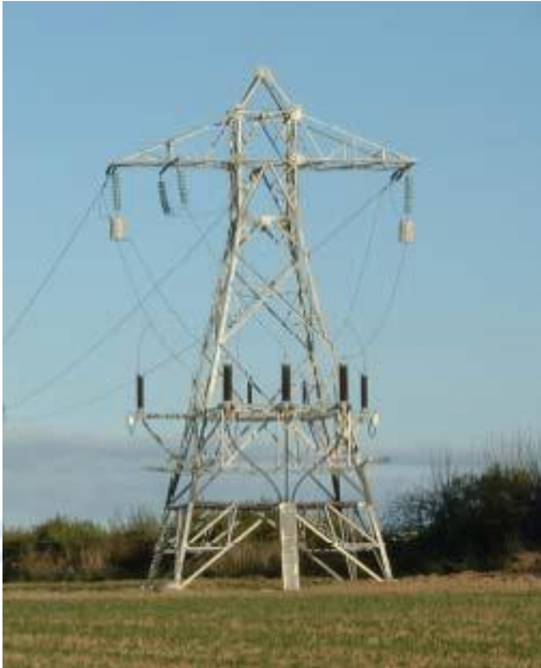
Figure 2: Terminations mounted on a platform on a 110kV overhead line tower
